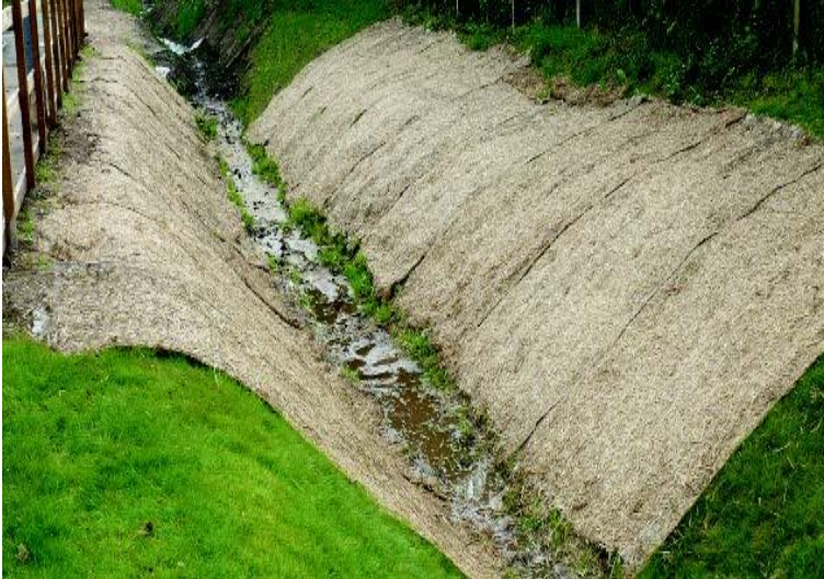
Figure 10-4 - Erosion Control Blanket
